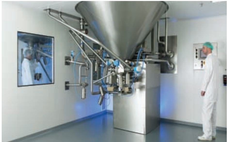
Vacuum processing: Lower floor section of the FrymaKoruma Dinex system at ASM, Switzerland
