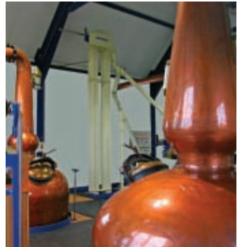
A Guttridge bucket elevator framed by the copper stills used in the whisky distilling process
